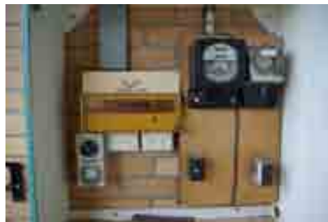
40) Backing to switchboard may contain asbestos.
