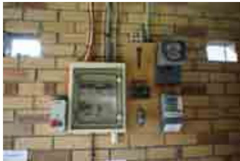
36) Electrical switch / meter board may contain traces of asbestos.
